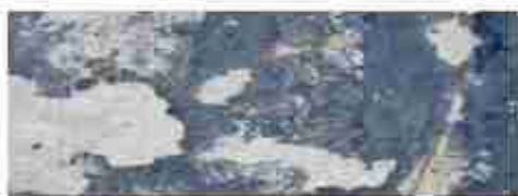
Geco Granite Crack Wall
